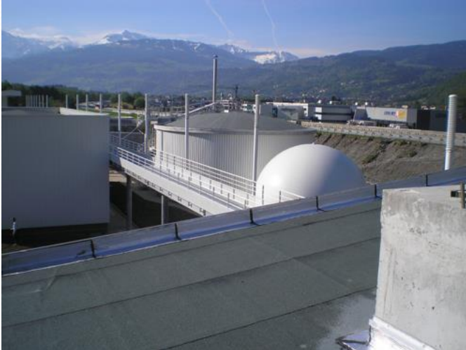
Station d'épuration du SIABS (source: SIABS)
